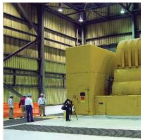
The turbine room at Palo Verde Nuclear Generating Station Unit 1, which set the record for most electricity produced by any nuclear power plant worldwide in 2009
